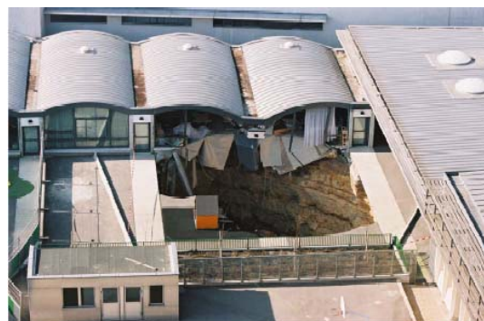
Example of a ground collapse in a school in Paris, where weak signals have been ignored
